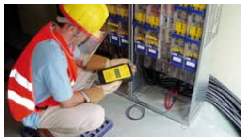
Cable identification in the LV output of an MV/LV transformer using the IC1G receiver (RX)
